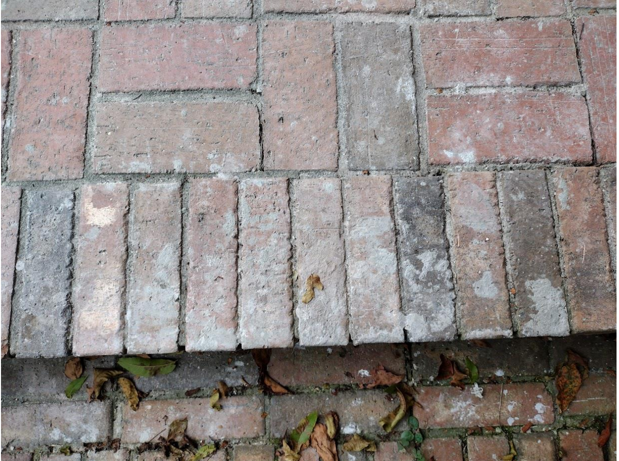
Thinset on brick porch, Photo 10.
