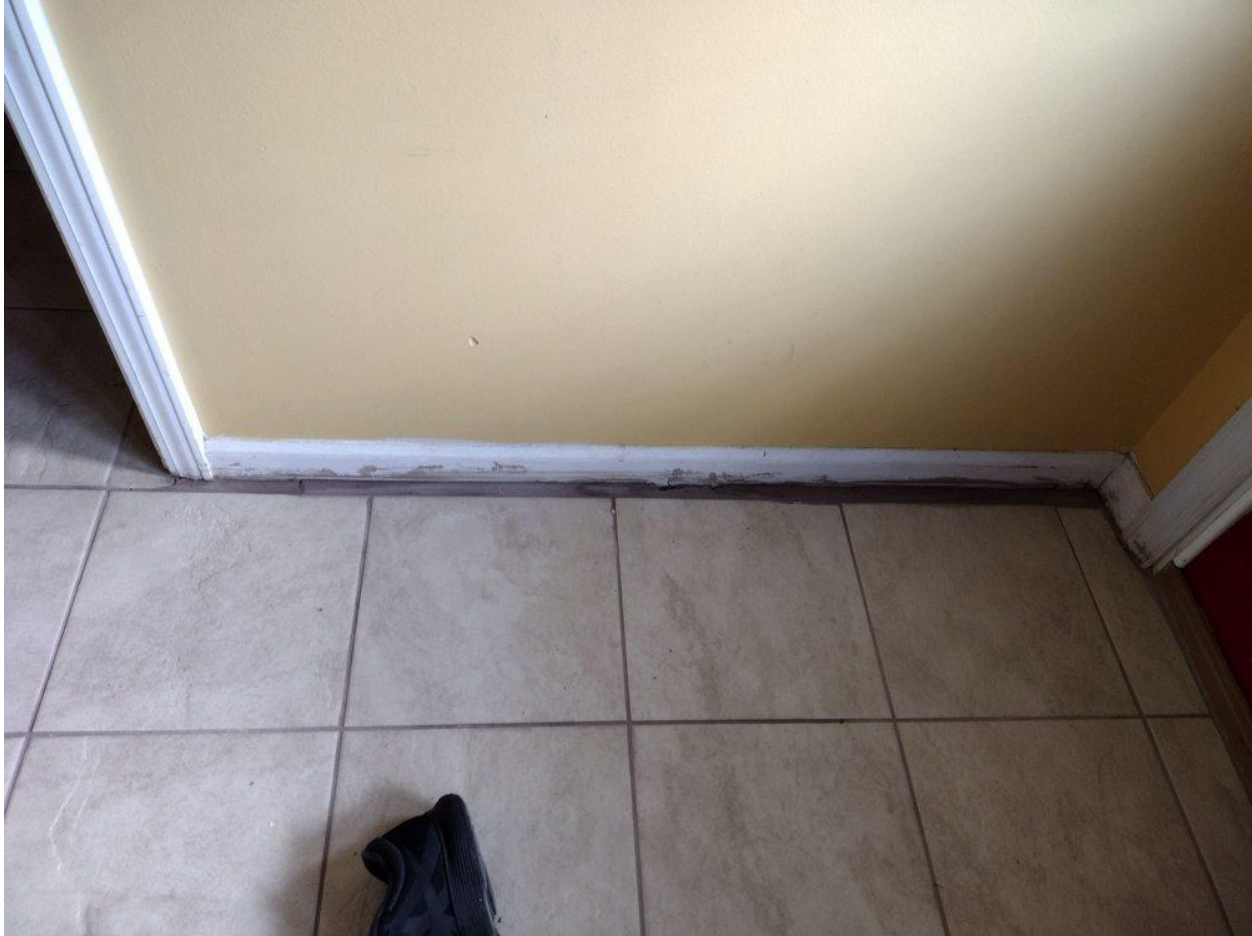
Grout on walls, Photo 5.
