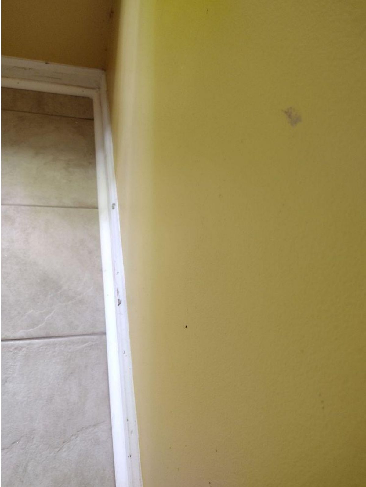
Grout on walls, Photo 6. Grout and thinset smeared on walls and baseboards.
