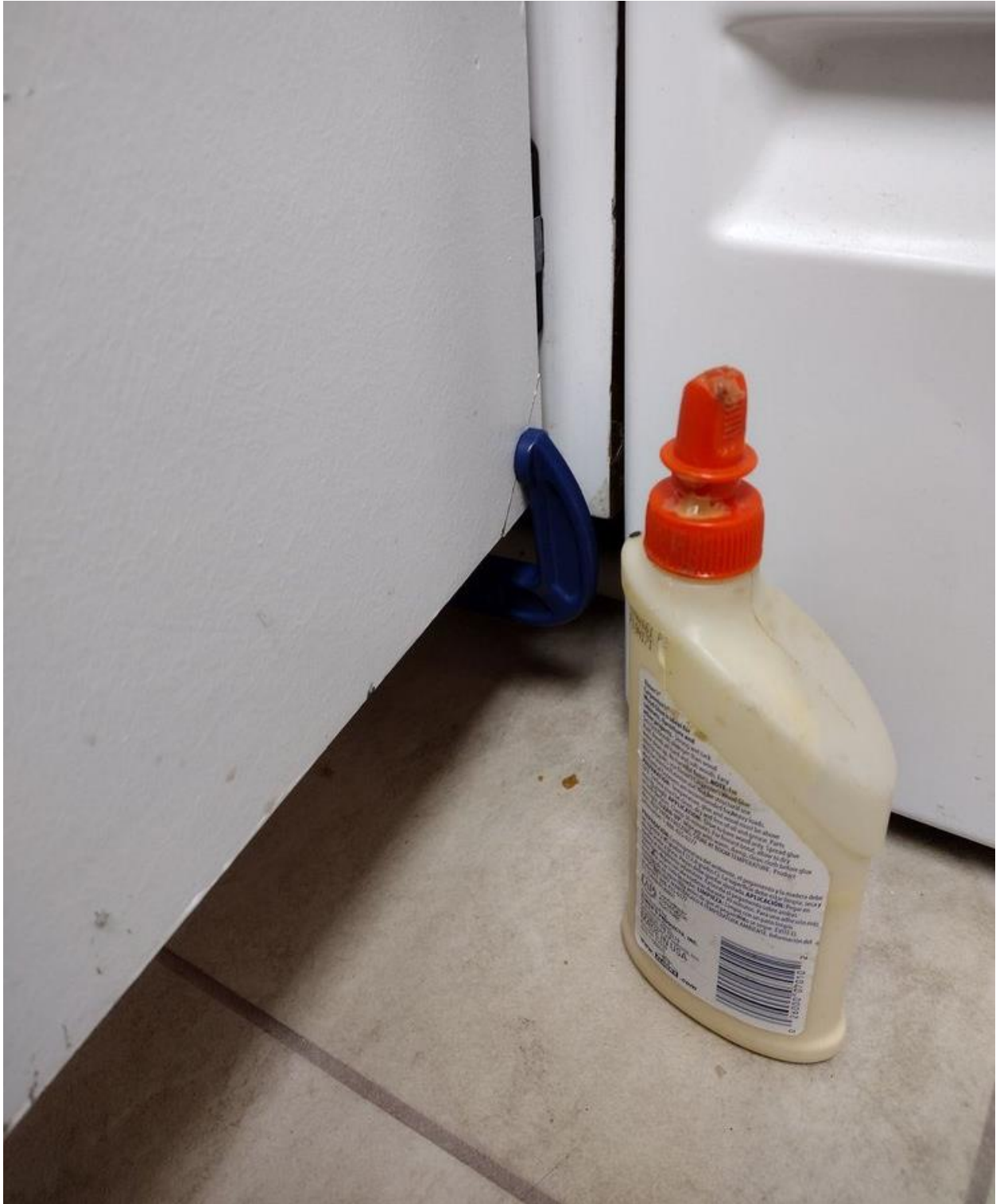
Broken kitchen cabinet, Photo 3.
