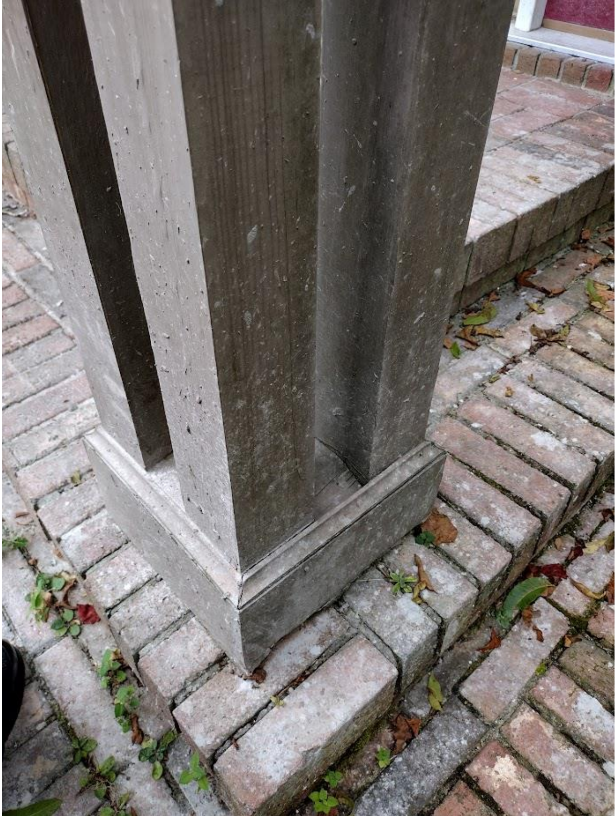
Thinset on brick porch, Photo 6.
